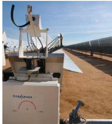
RSR system installed at CSP plant in California
