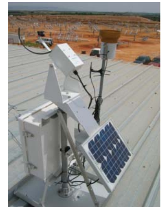
Rooftop mounted RSR system installed for PV/CSP plant developer in southern Spain
